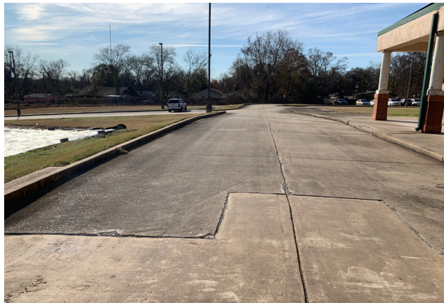
Galloway Elementary Pre-Installation Photo
