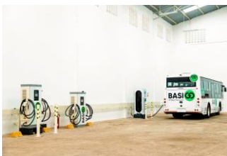
Figure 19: BasiGo bus at charging depot
